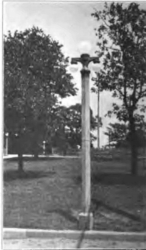
STILES PARK, SHOWING THREE-LIGHT TUNGSTEN POST, WITH ONE-LIGHT POSTS IN THE BACKGROUND
